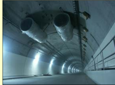
Jet Fans in Main Tunnel
