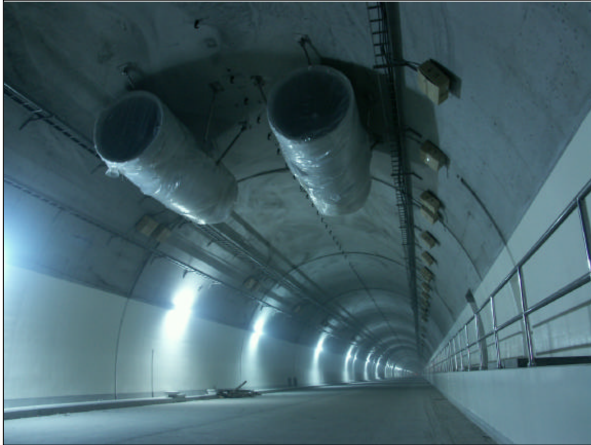
Jet Fans in Main Tunnel
